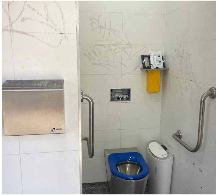
Figure 13: Newly completed Frankston Station public toilet, unavailable due to vandalism
